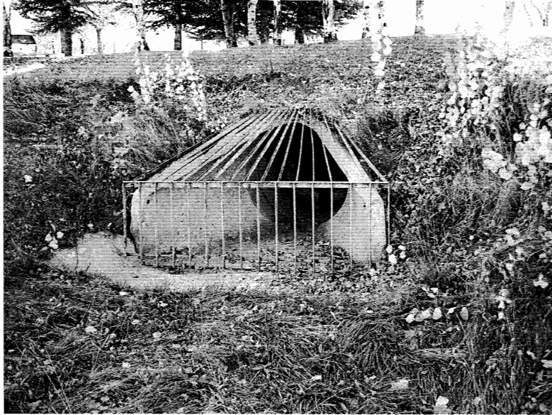
Inlet pipe with trashrack
