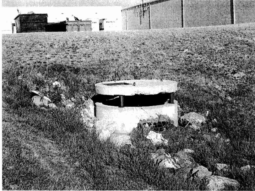
Outlet capacity - maintenance
