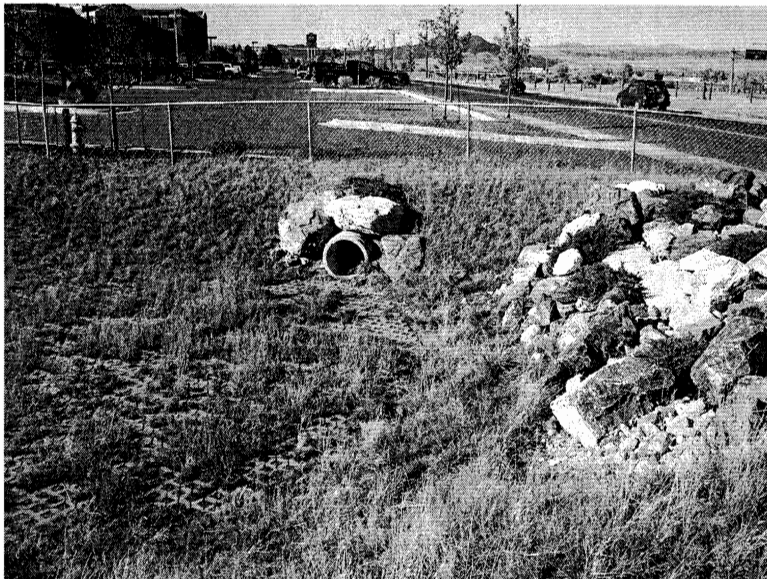
Outlet capacity - pipes with fence
